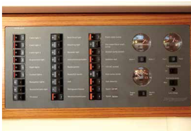
The custom-designed electronic control panel
