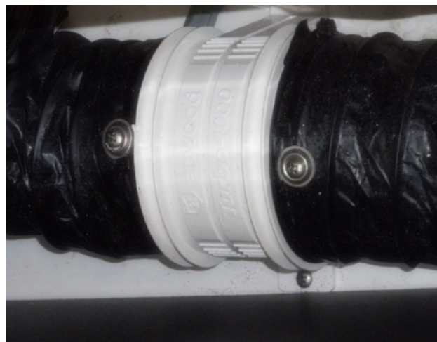
Typical Ventilation Blower with Hose
