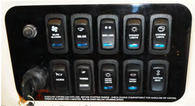
Typical Switch Panel Shown
