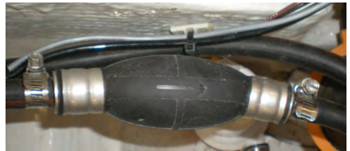
FUEL PRIMER BULB IN SUMP AREA
