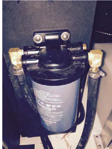
CHECKING IN-LINE WATER SEPARATOR FILTER
