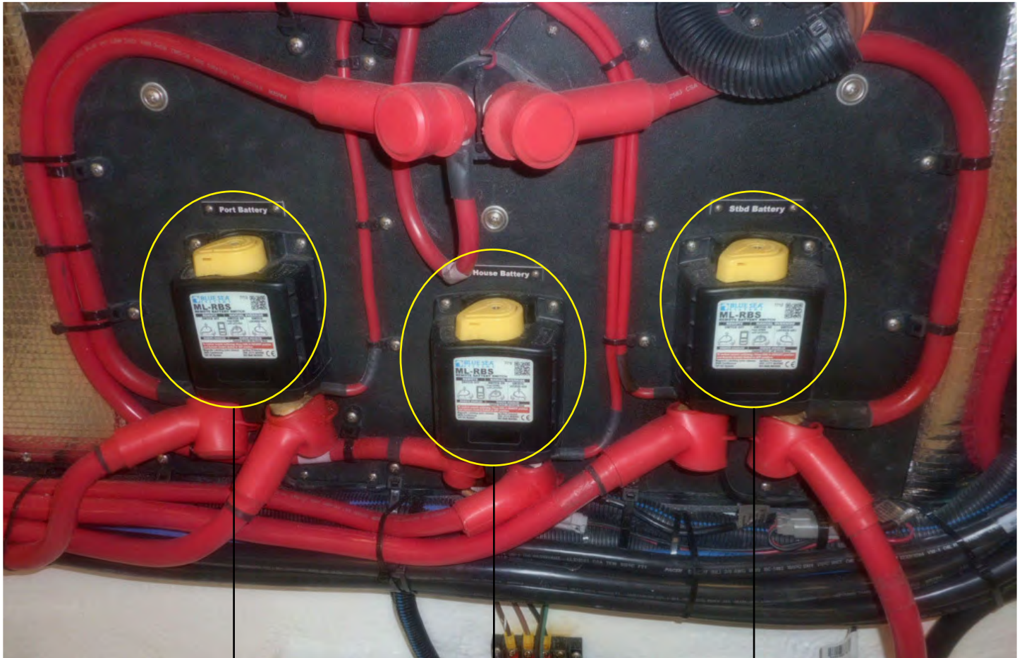
PORT REMOTE BATTERY SWITCH
