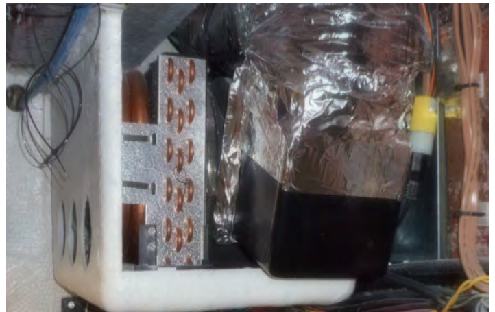
STARBOARD AC UNIT
