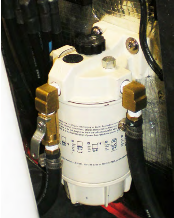
DIESEL GEN-SET PRIMARY IN-LINE WATER SEPARATOR FILTER
