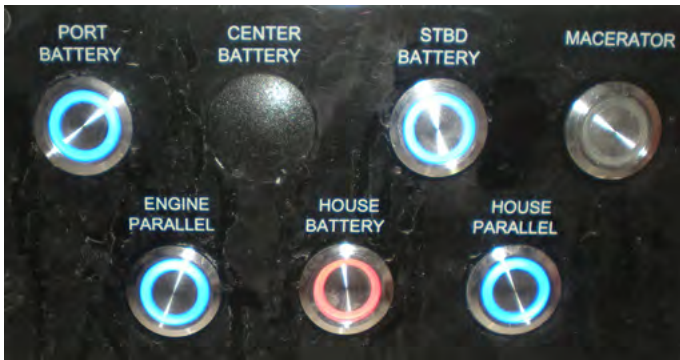
TYPICAL EARLIER BATTERY ACTIVATION PANEL
