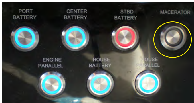
BATTERY ACTIVATION PANEL
