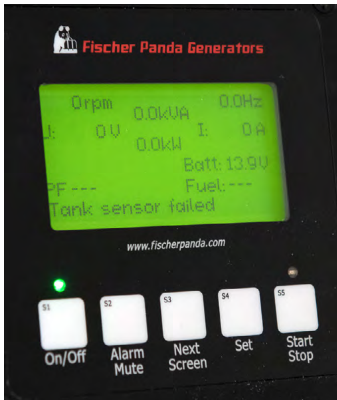
DIESEL GENERATOR DISPLAY PANEL
